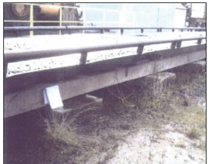
Figure 2: Side rail and drop off.
